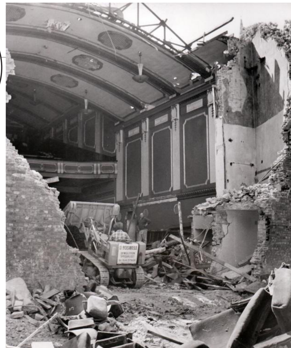
St George's Hall being demolished by contractor, Dennis Boswell. Source: York Press.
