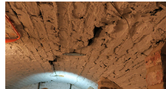
East Cellar, Structural Crack to Ceiling.
