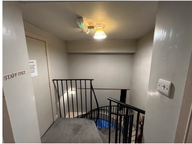
Left to Right - Second floor spiral stair landing; Corridor looking East; Kitchenette; Hall between Office and Kitchen.
