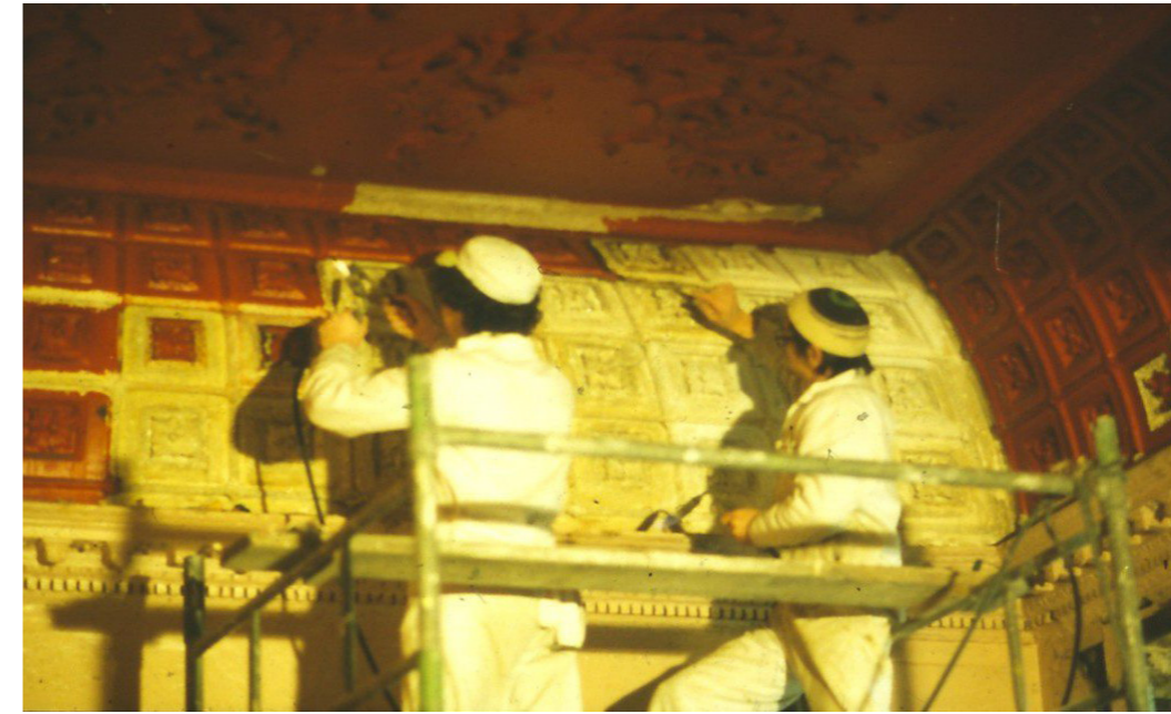
Bellerby's (Painting and Decorating) carrying out work to remove many layers of red paint applied during Cinema ownership, c.1982. York Civic Trust Archive.
