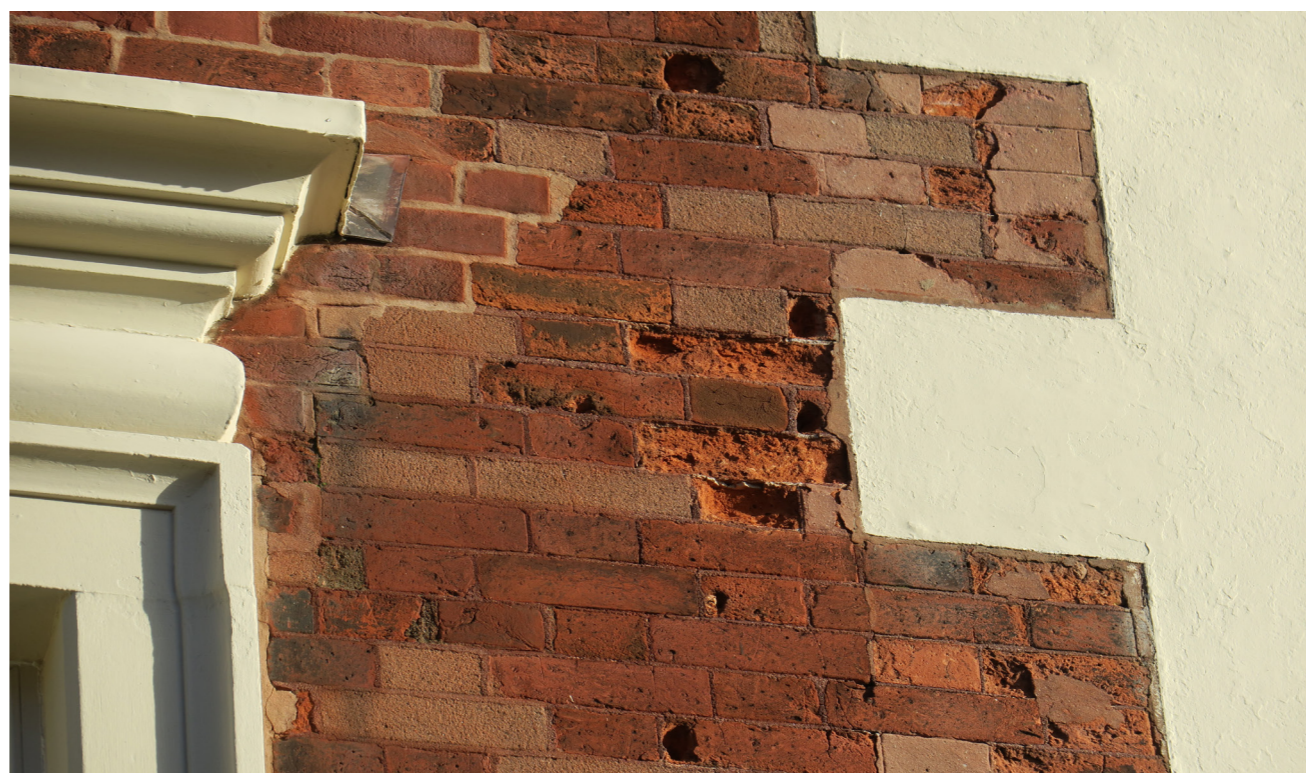
View of decay to existing frontage.
