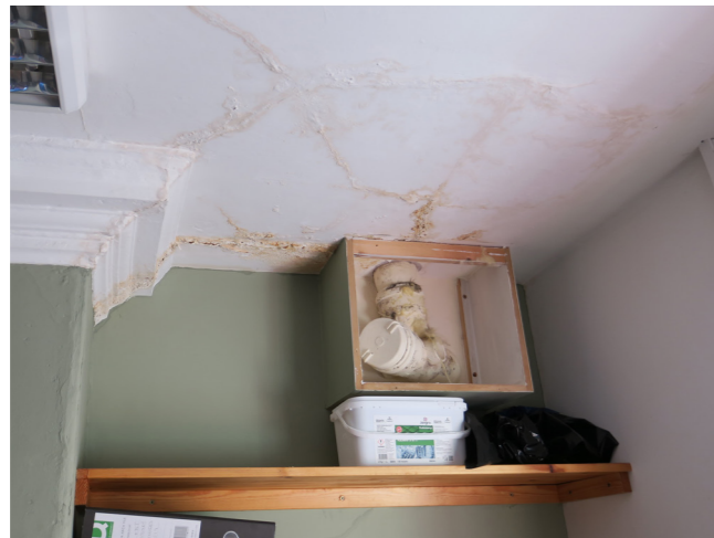
East Archive Room, Leak to South-East Corner of Room; Cracking to Ceiling near door; Bathroom - West Elevation; East Elevation.
