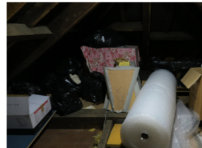
Attic 2, North area has no accessible floor.
