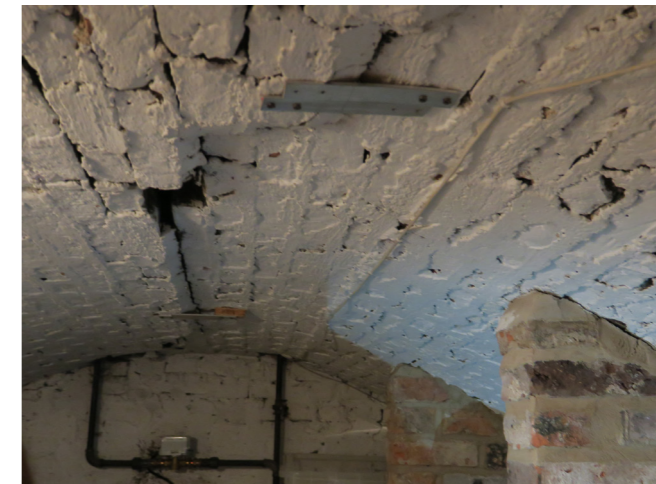
East Cellar, Structural Crack to Ceiling.
