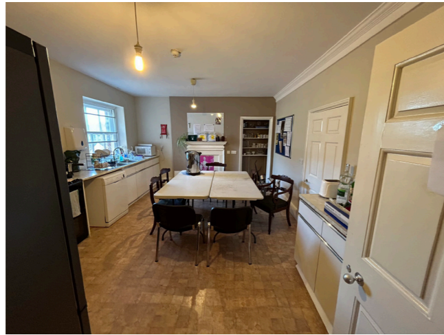
Kitchen - East Elevation; North Elevation; West Elevation; Hairline Fractures to Ceiling.
